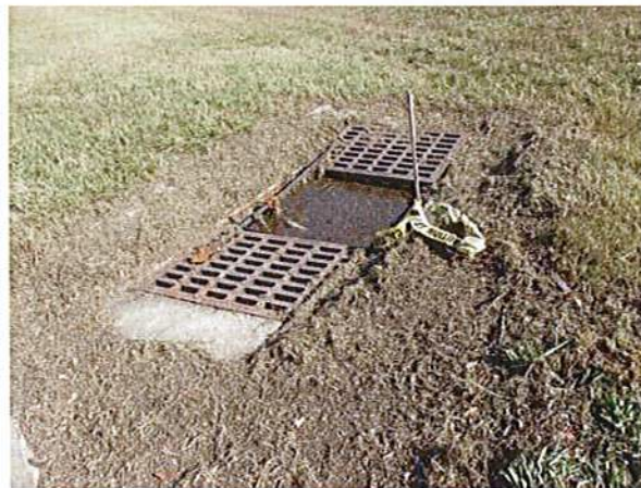
Ditch bottom inlet control structure with missing grate
