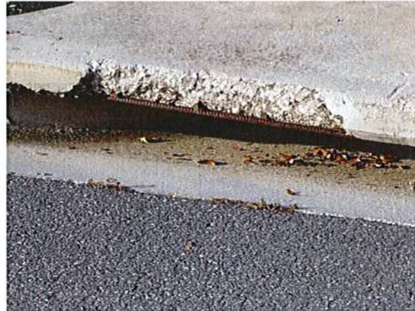
Damaged catch basin
