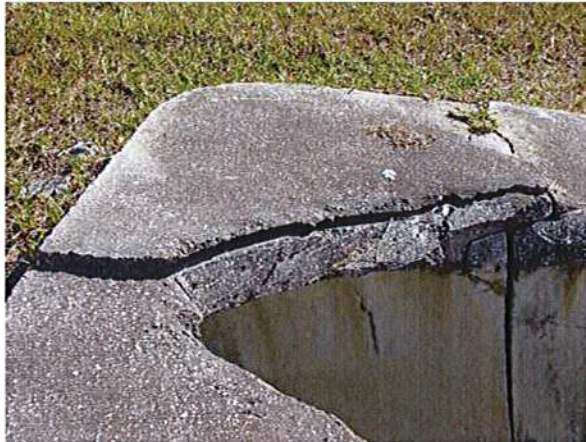
Damaged mitered end section control structure
